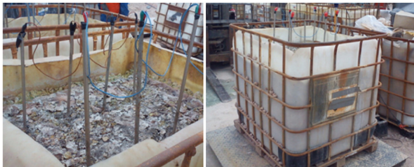
Fig. 5. Photograph showing the tanks used in the pilot tests of electroosmotic drainage in operation, the linear distribution of the electrodes and verticality of their positioning.
